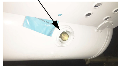
Propane Tank Features -Typical View
