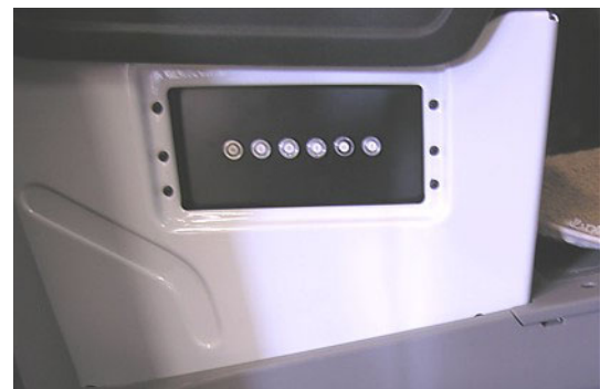
Automotive Chassis 12-Volt Circuit Breakers Located on outboard side of passenger seat (Shown with cover removed). -Typical View
