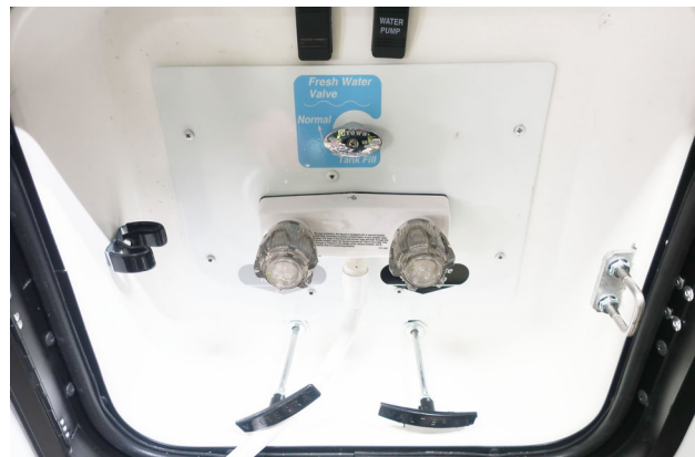
Exterior Shower/Wash Station (524T and 524R) -Typical View
