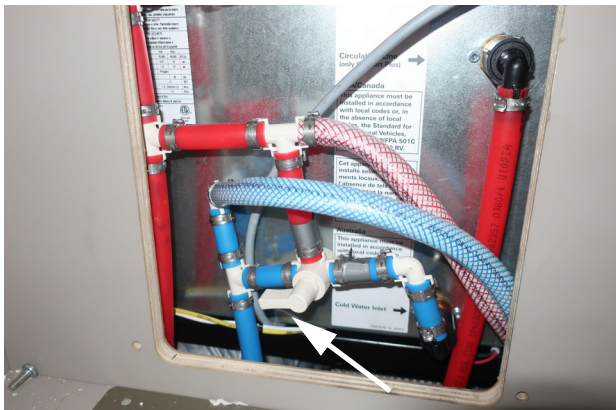
Winterization Valve #1 Water Heater Bypass on model 524R located inside the galley. (Shown in Normal position). -Typical View
