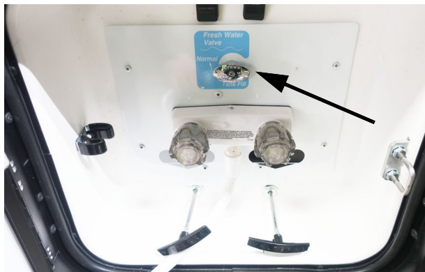
Fresh Water Valve (Located in water service center) (524T and 524R) -Typical View
