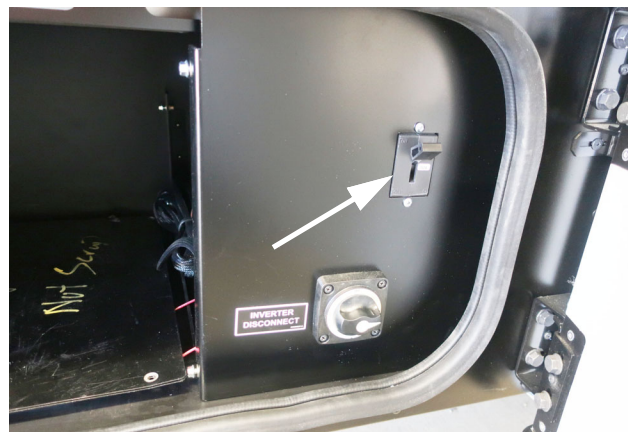
250 Amp Circuit Breaker (Located in the passenger side compartment) (Options 52D 78G shown) -Typical view
