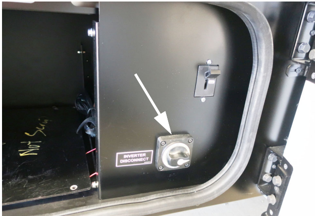
Inverter/charger disconnect switch. (Located in the passenger side compartment) (Options 52D 78G shown) -Typical view
